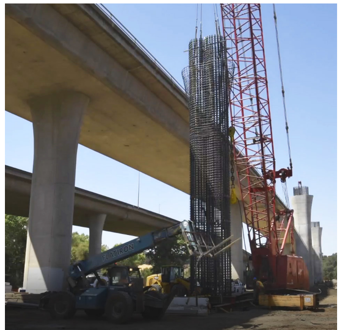
Construction Crews constructing 60-foot columns to support the third lane on Highway 65
